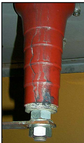
Fig. 2. Heavily tracked generator bushing
